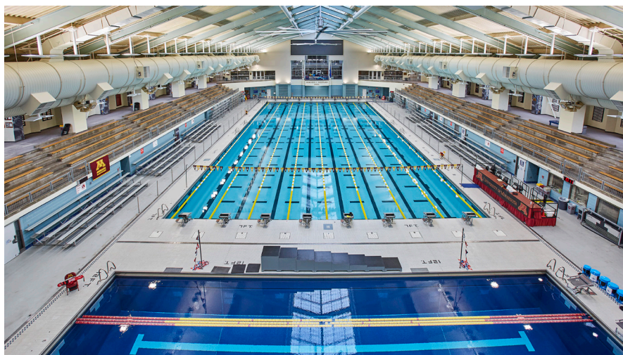
Healthy and durable pool spaces require proper air distribution to all space micro-zones. Zones shown here include swimming, deck, and elevated spectator areas, and exterior-facing glass, wall, and roof areas.
